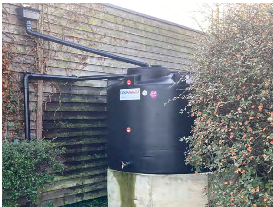
Rainwater harvesting in Woodford Park
