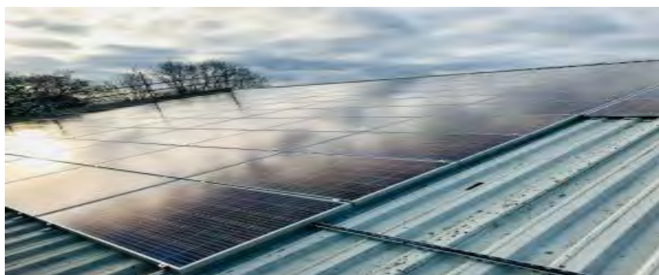
Solar panels on Woodford Park Leisure Centre
